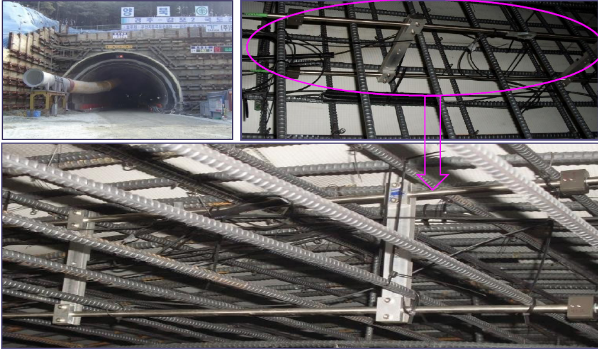
Ways to measure the deformation of the tunnel after installing two 1000mm strain sensors in parallel.
